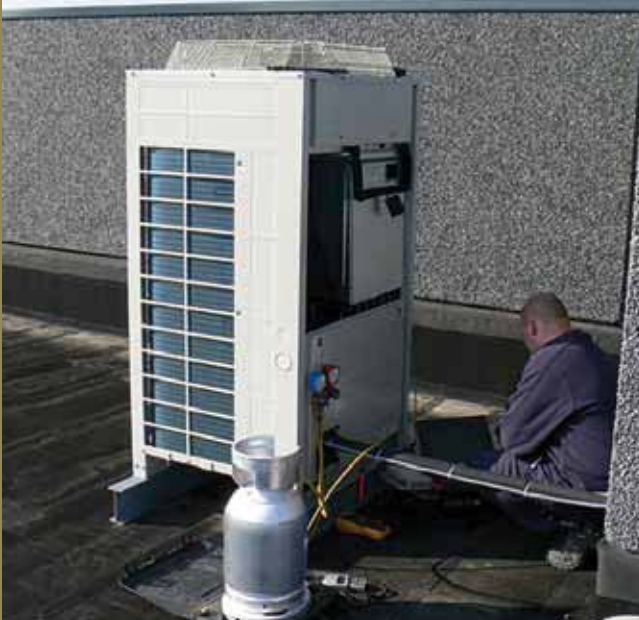
➤ Daikin Belgium and Luxembourg technician inspects refrigerant charge during maintenance.
